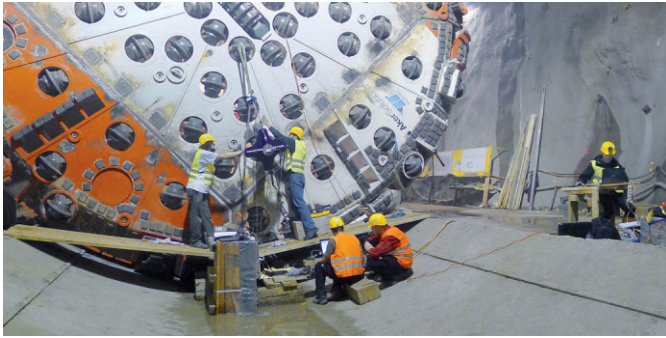
Fig. 5. Calibration test in the assembly cavern of the first Koralm Tunnel TBM
